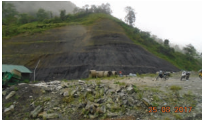
Upstream slope of national highway - landslide damage
