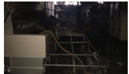
Factory building, machinery and electroplating line - fire damage
