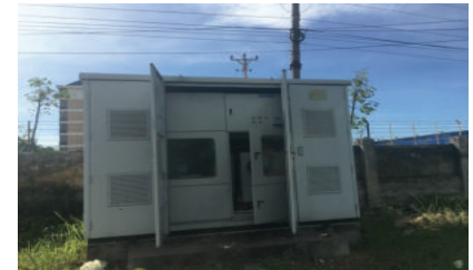
560kVA substation damage
