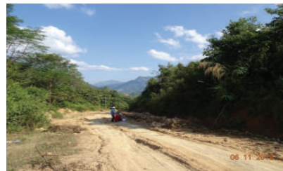
Road pavement - landslide damage
