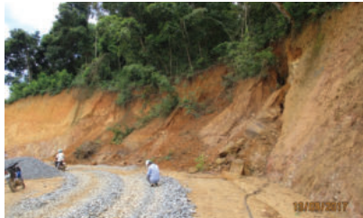
Slope and drainage culvert - landslide damage
