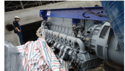
Standby generator - drop damage
