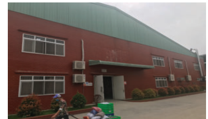
Factory building, machinery, equipment and goods - fire damage
