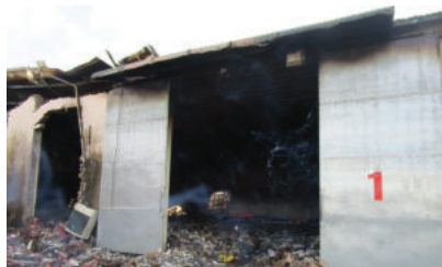
Bonded warehouse - fire damage
