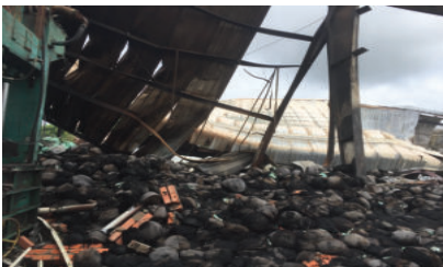
Warehouse - fire damage
