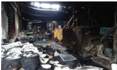
Factory building, machinery and goods - fire damage
