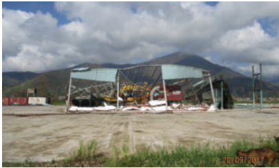
Factory building, machinery and goods - storm damage
